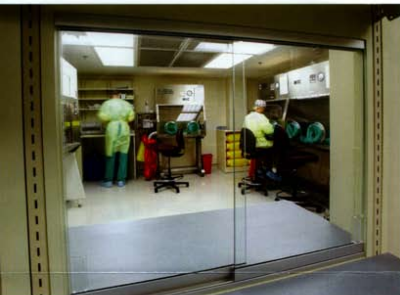
Buffer Area with Barrier Isolation Technology
